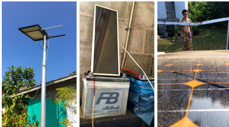
Figure 1: A broken SHS, a 'fixed' SHS and the school's neglected solar system
