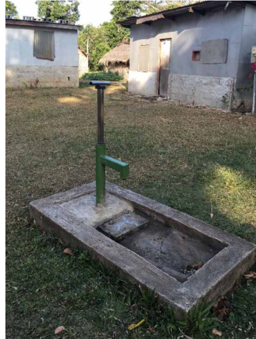
Figure 7 | Example of a Nira AF-85 pump stand encased in concrete.
