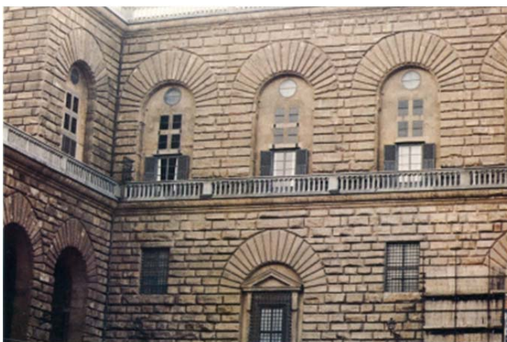
Figure 32. Pitti Palace, Florence. Some parts of Pietra Forte restored with Fomblin YR (1982-87) [17 [1]].
