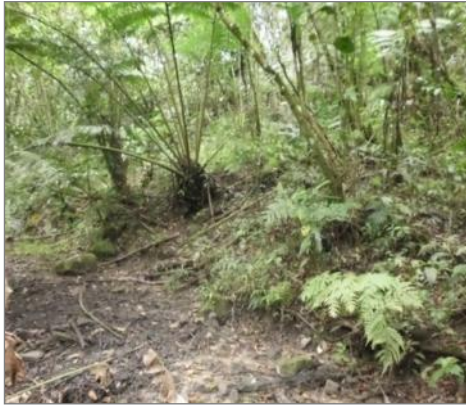
Fig. 84 Degraded terrace due to erosion processes at site M28-0010 (SK)
