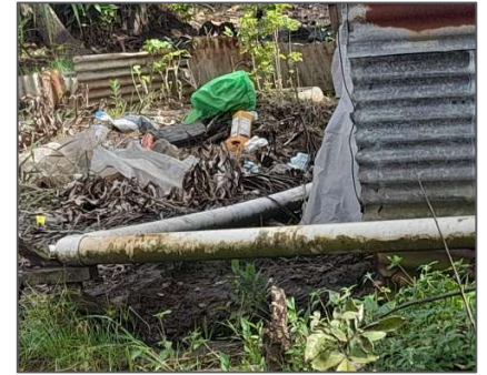
Figure 11: Exposed sewerage pipes
