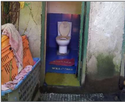
Figure 9: Superstructure and latrine showing water level encroachment of water (dark water marks on right)
