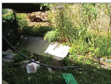
Figure 2: Exposed water pipes
