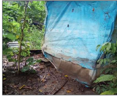
Figure 10: Substandard superstructure materials
