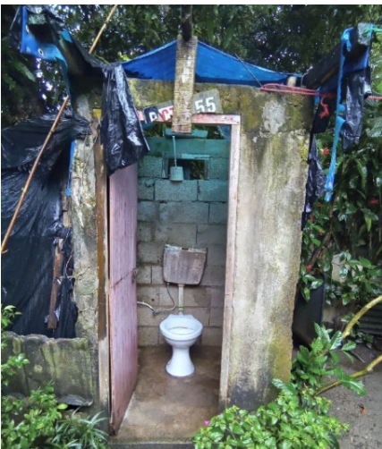
FIGURE 1: RESIDENT'S TOILET IN INFORMAL SETTLEMENT IN PORT VILA
