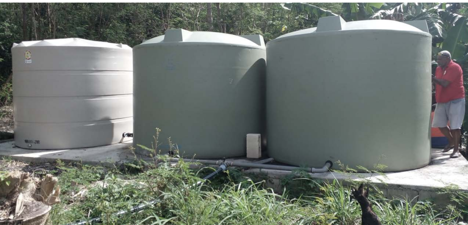
Image: Storage tanks, Lelepa (w/ Denny Manvoi, VRC)
