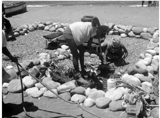
Local school children have selected salt tolerant plants and planted them into the beach level wetland that is now treating sewage and wastewater from communal showers.
