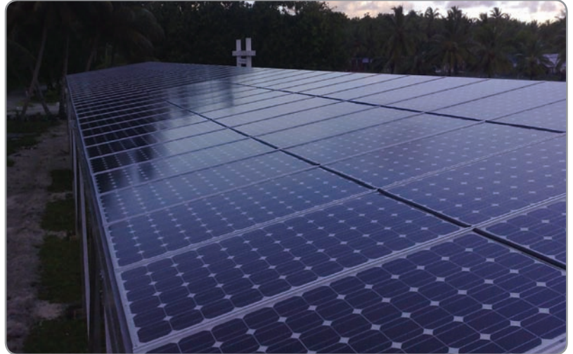
Figure 5: Solar panels on grandstand roof at the Motufoua School Stadium
