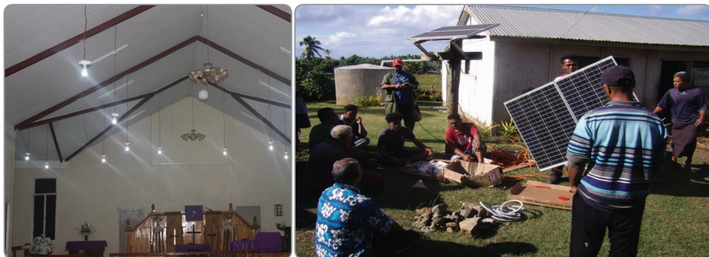
Figure 4: (Left) Well-lit church in Mo'unga'one, (Right) System installation
