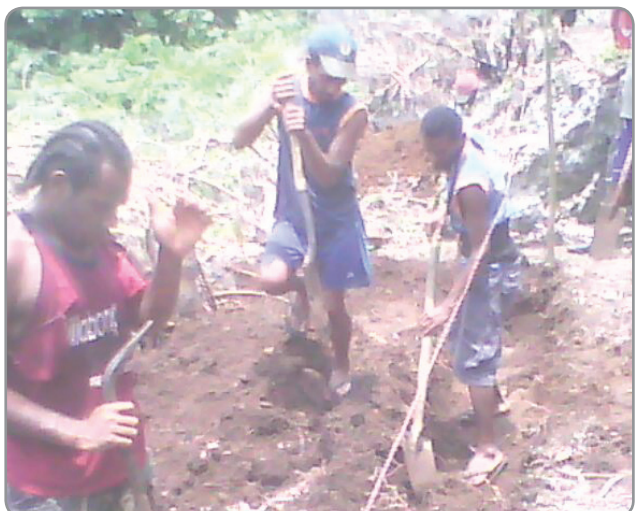
Figure 11: Digging the trench for the Talise hydropower system (Photo taken in November 2011)
