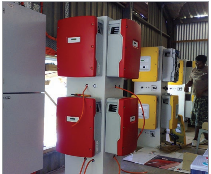
Figure 6: Battery banks and inverters.
