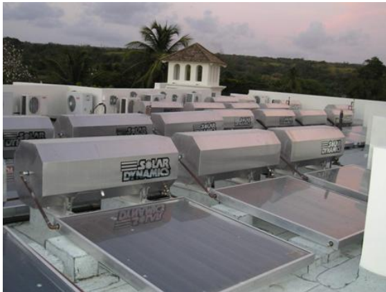
Figure 12: Solar Water Heater
