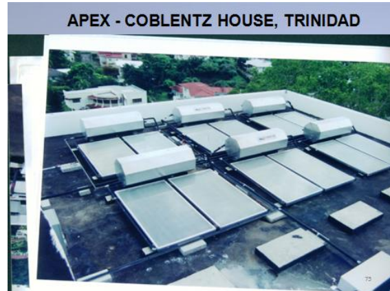
Figure 13: Solar Water Heater
