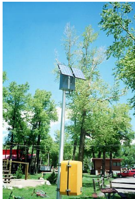
Figure 5: PV-powered Flood gate Controller
