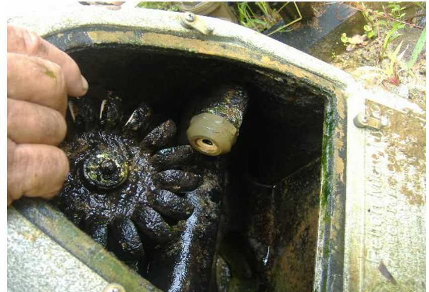
The turbine used at Tiko's nano-hydro system
