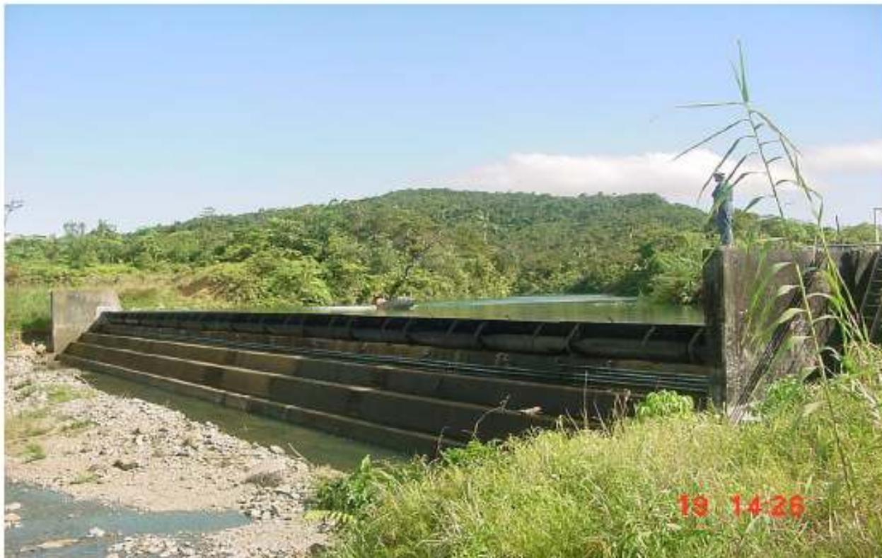
Wainisavulevu Weir with Rubber Dam
