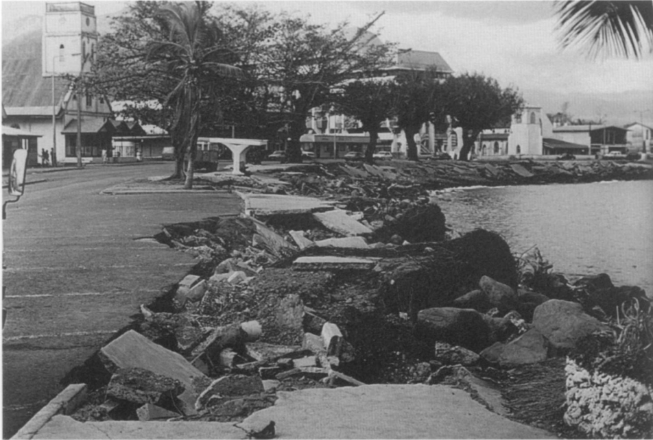
Figure 5. Damage to the seawall at Apia, the capital of Western Samoa, caused by storm waves associated with Tropical Cyclone Ofa in 1990. Many seawalls in the Pacific islands exacerbate the problems they are intended to solve; many are of an entirely inappropriate design and construction.
