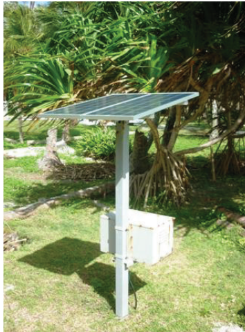
Household solar panel in Arno Arno Village, Arno Atoll, Republic of the Marshall Islands
