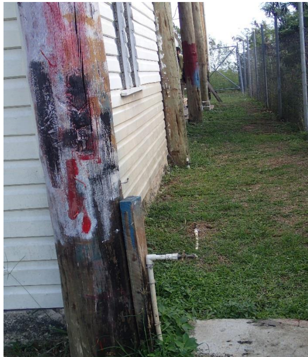
H. Hand washing facility outside the building
